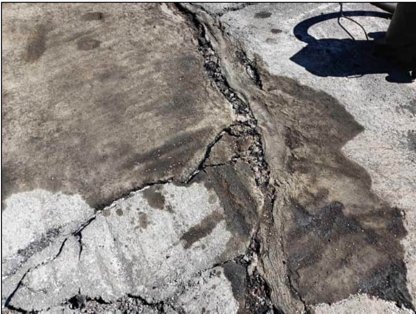
Crack in Pavement Creates Pathway for Oil to Impact Soil Below
