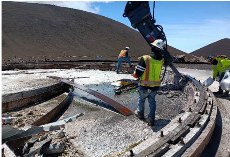
^ 10:56am - spilled oil on concrete
