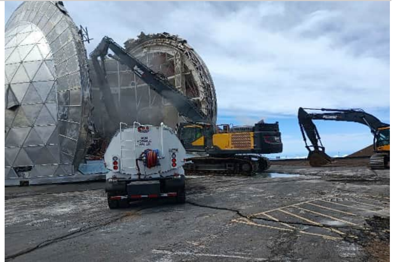
^ 10:34:05am - oil spilled from excavator
