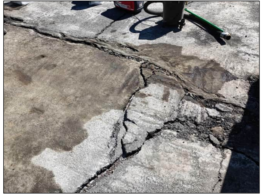
Staining Remains Post-Clean Up
