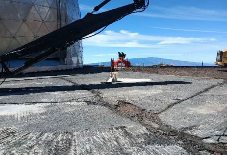
^ 10:45am - cleaned up oil leak
