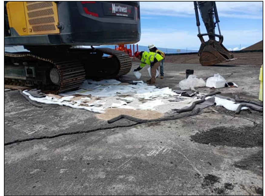
Applying Absorbent Pads to Spill on 4/30/2024
